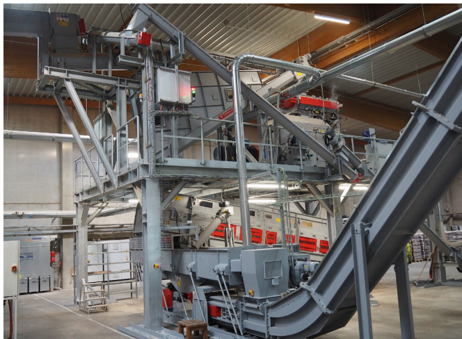
Compact, high-performance plant: above the pellet press, below the cooler and the vibrating chute into the silo
