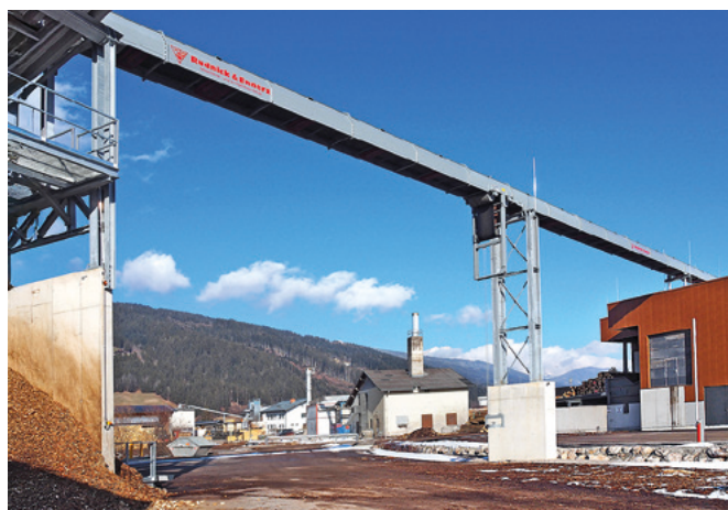
A tubular belt conveyor transports the optimally shredded wood waste from the log yard (right) to the biomass heating plant
