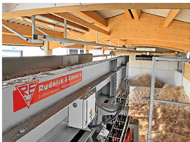
Controlled infeed of the homogeneous material to the heating plant – either into the crane's loading bin or automatically into a pre-bin
